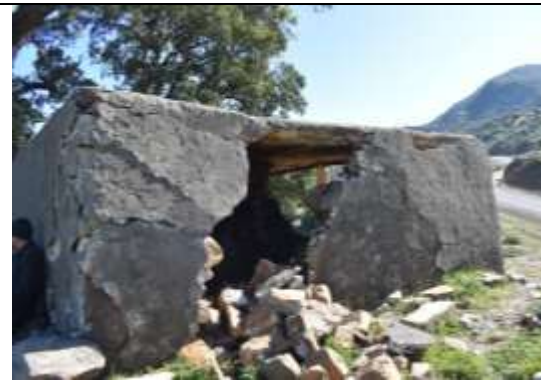
Image 5. The deterioration of the shrine of Sidi Lahcen
